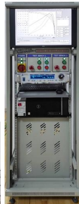
CONTROL AND REGULATION RACK
